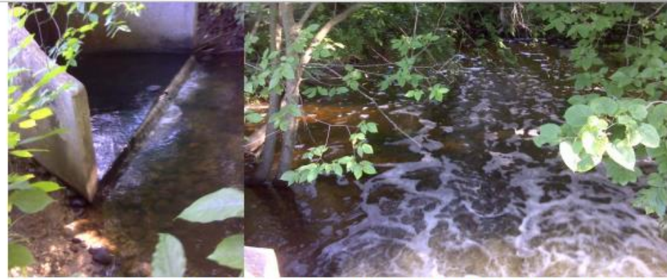
Figure 37: Unnamed Creek culvert outlet on County Road 14 on July 2, 2013, and July 18, 2013 after heavy rainfall.
