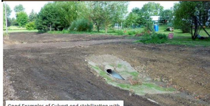
Good Examples of Culvert end stabilization with Category 25 blanket, following the pictorial drawing above.
